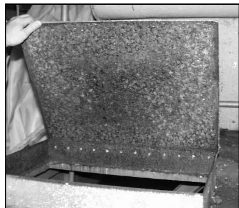
Cleanout Hatch Shows Machine is a Rainmaker
